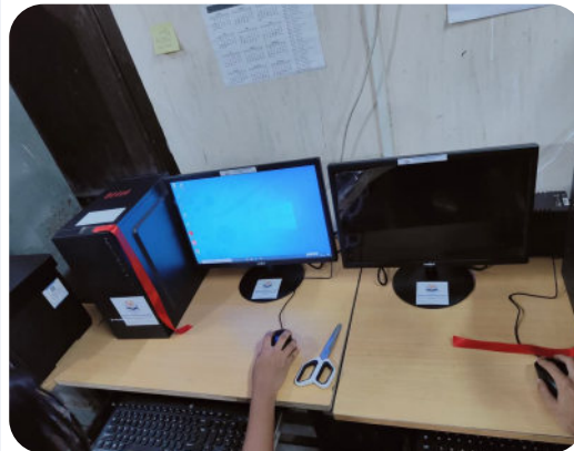
The installed desktop computers and UPS
