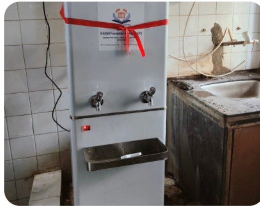
One of the water coolers installed in the Mumbai Veterinary College
